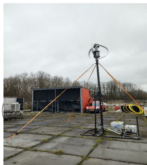
Figure 1: 300 W HI VAWT TECHNOLOGY CORP.
